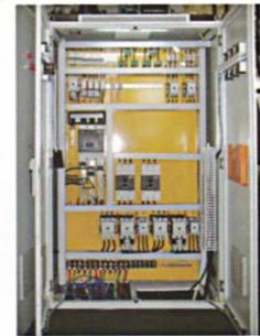
威图控制柜 Rittal control cabinet
